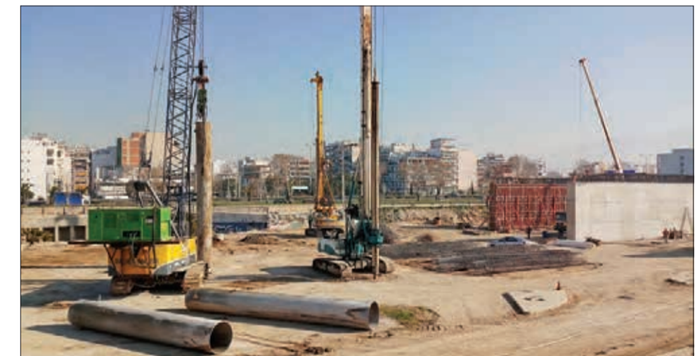
Infrastructure work for the rehabilitation of Piraeus in the region of Attica
